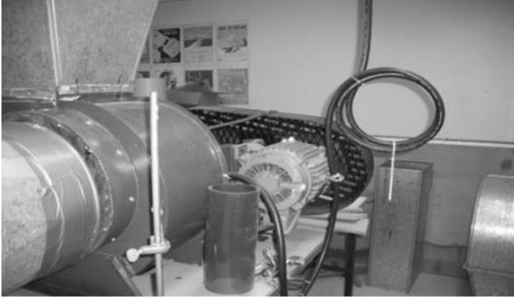
Figure 78: Buffalo Load fan belt transmission
