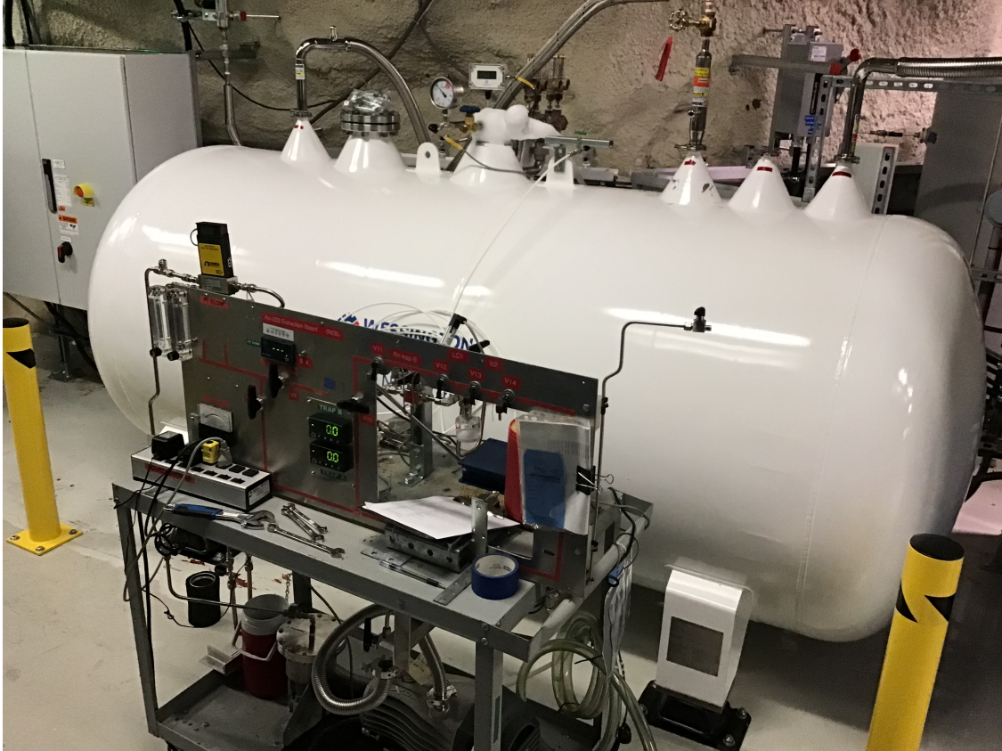
Figure 4.5: Underground LN 2 Plant.
