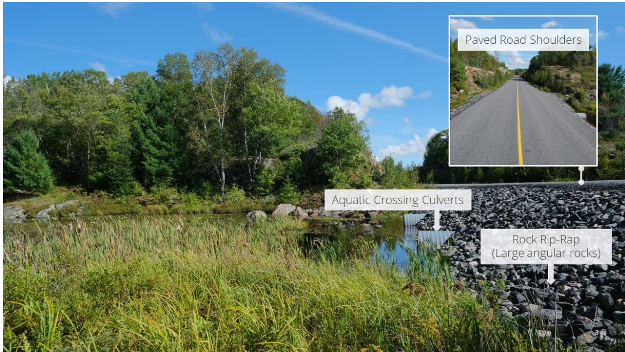
Figure 1.2: Example photo of the mitigation design at study site number 3 (refer to Figure 1.1), showing upgraded culverts, rip-rap on road embankments, and the paved road including road shoulders.
