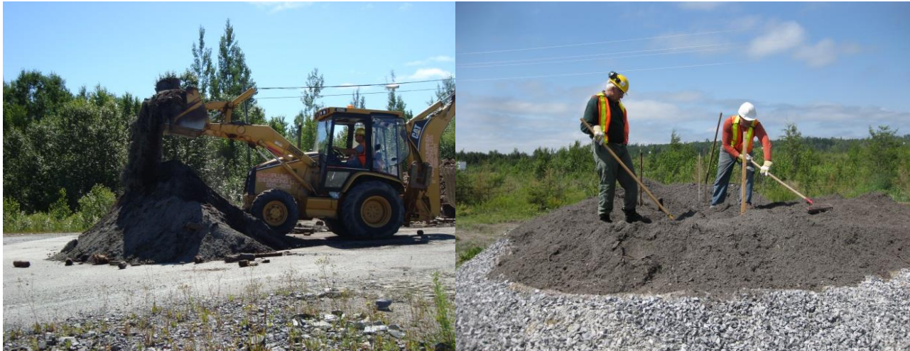
Figure 30. Technosols for each cell were produced independently. (L) Finely crushed waste rock and wood waste were combined in volume ratios using a backhoe to yield desired soil. (R) Technosols were deposited on to field lysimeter cells and hand raked to 30 or 60 cm thickness.
