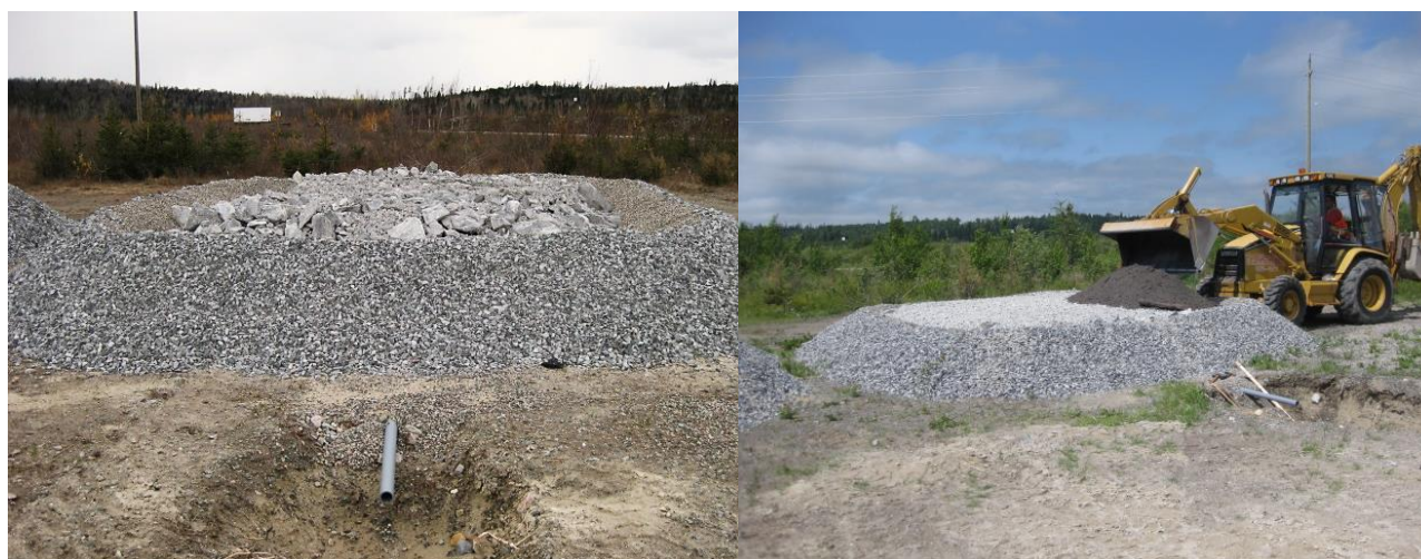
Figure 29. (L) Base of a reclamation plot, showing the front drainage tube to collect percolation waters. (R) Depositing a Technosol on the top of the reclamation plot.
