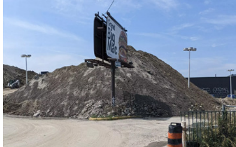
2022 - Large mounds of dirt appear from off-site excavation, and pose as a health risk to the community.
