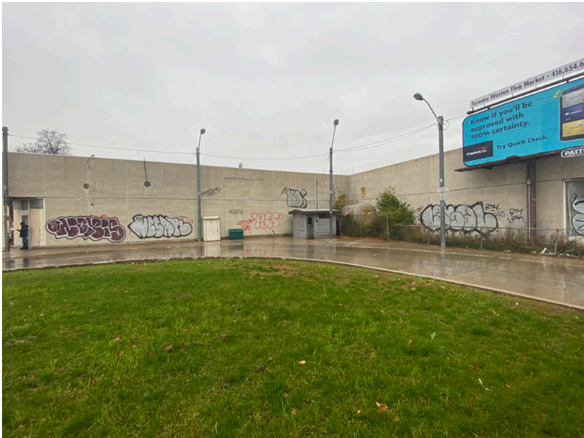
Figure 49: Exterior View of Bus Turnaround and Building Dilapidation.
