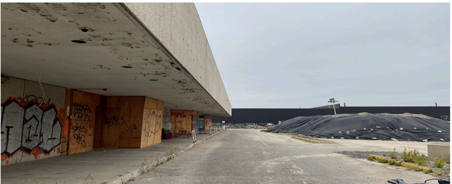
Figure 48: Exterior Photograph of the Parking Lot showing boarded-up walls and potential windows on the South facade.
